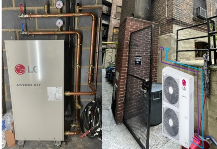
Figure 6. Close up image of indoor Hydro Kit module and outdoor heat pump unit with a proposed schematic of how units would be floor mounted at a rear wall of a typical multifamily building Source: Steven Winter Associates 2024.
